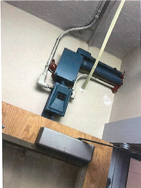
Random circuit breakers mounted in stairwell
