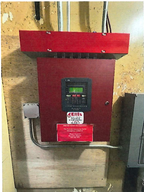
Fire alarm control panel
